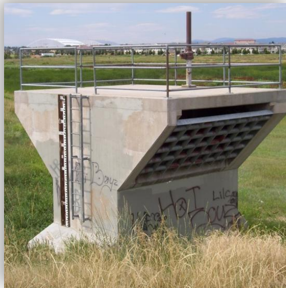
Right: the tall overflow tower houses a 60-inch pipe to take away large loads of water.
