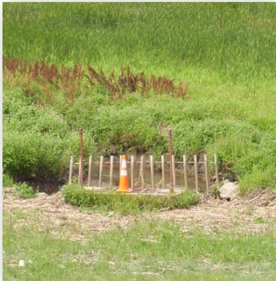
Left: the Trash Rack Grate, located nearly 75 yards southwest of the Tower Structure, plugs up easily with debris. The cone in the picture is resting on the overflow grate.
