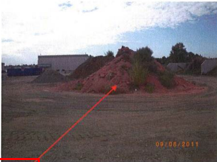
Zone 2 Bulk stockpiles observed not covered or contained Photos #23
