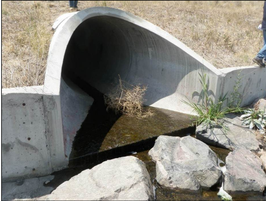
Photograph 9. View of outfall to Tollgate Creek located to the northeast of Victor Street and Fitzsimmons Parkway. Note the dry weather discharge actively flowing from the outfall during the inspection.
