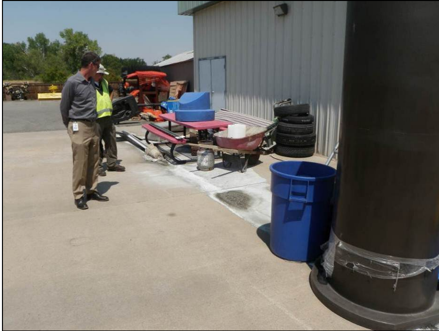
Photograph 19. View facing northeast at stain of unknown substance on the impervious surface to the west of the Parks and Recreation Storage building at the Central Facility. Note the lack of spill response BMPs implemented.
