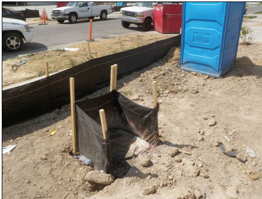
Photograph 4. View facing northwest at the active construction site for the Lennar Homes development. Note the use of an effective and innovative BMP to prevent concrete washout from discharging from the site.
