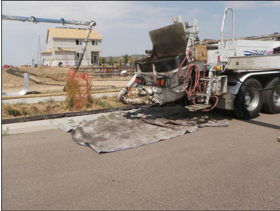
Photograph 1. View facing north at staging area for construction-related activities at the DR Horton at Traditions new development. Note the effective use of ground cover to protect the impervious surface from exposure to construction materials.
