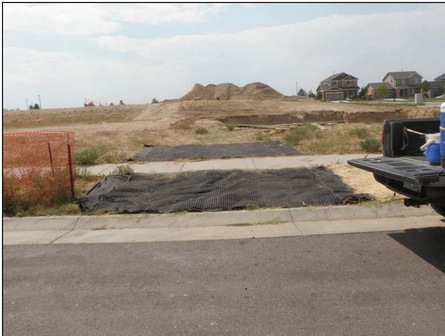
Photograph 2. View facing north at an active construction site for the DR Horton at Traditions new development. Note the effective use of plastic to protect the pervious surface from construction vehicles and prevent sediment drag-out from entering the roadway.
