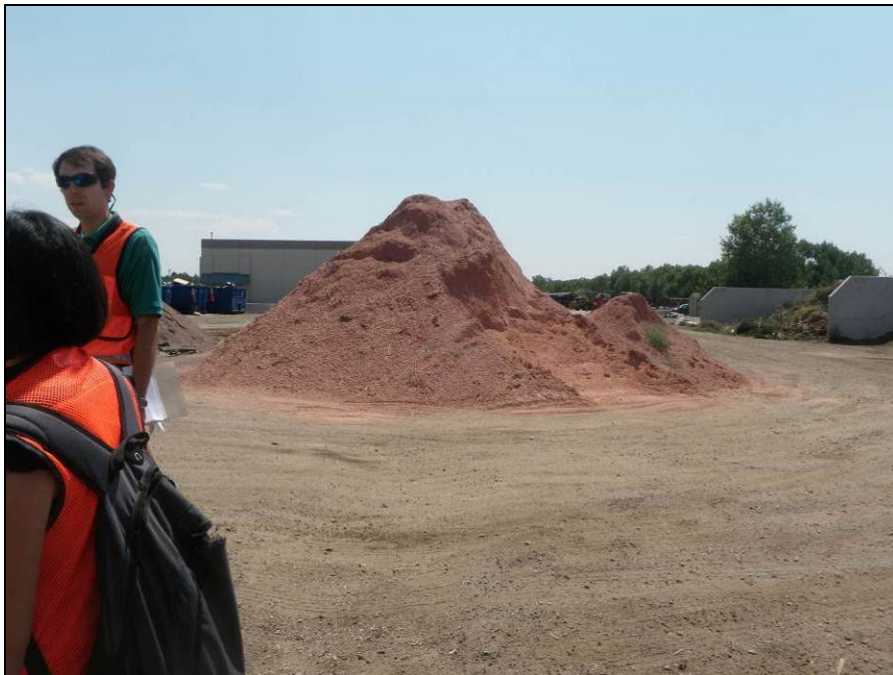
Photograph 20. View facing south at pile of stored landscaping material at the Central Facility. Note the lack of erosion and sediment control BMP implementation.
