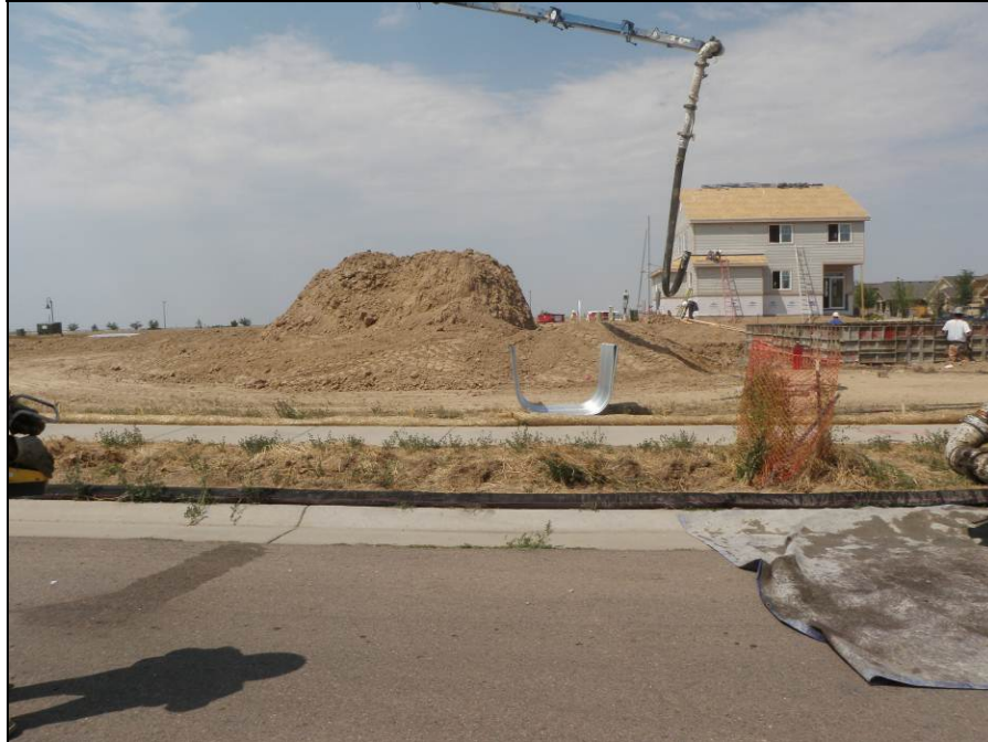
Photograph 3. View facing north at the active construction site for the DR Horton at Traditions new development. Note the use of straw bales along the curb to protect sediment drag-out from entering the roadway. In addition, the perimeter of the materials stockpile has been compressed to prevent the mobilization of sediment.
