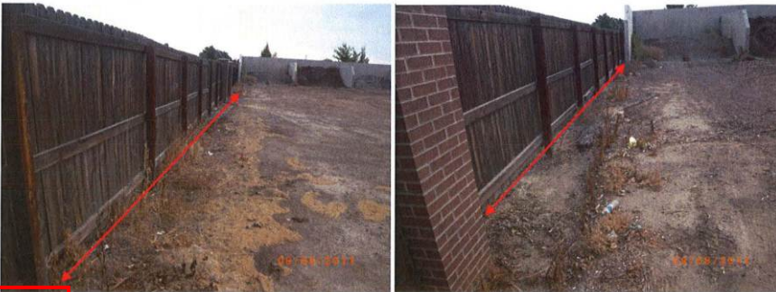
Zone 4 In 2010 straw wattle was installed at the west end of the northern property line for sediment control and stockpile protection. That protection has been removed. Photos #19, 22
