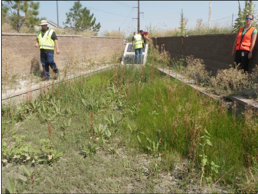
Photograph 7. Close-up view facing north at the the detention and water quality pond outfall at the Southlands Self Storage.
