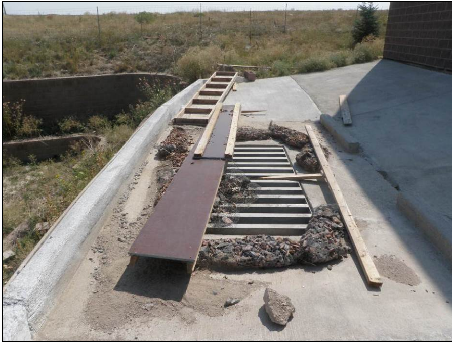
Photograph 5. View facing east at the stormwater drain leading to the detention and water quality pond at the Southlands Self Storage. Note the accumulation of sediment and construction debris that has not been removed.
