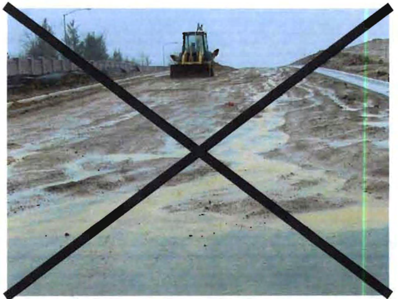
Unpaved, temporary or haul roads can easily erode when no control features are installed.
